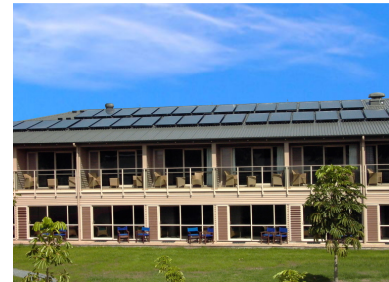
Largest single flat plate collector system in New Zealand (2007), 106m 2 Installation on the Millennium Copthorne Hotel and Resort, in the Bay Of Islands.
